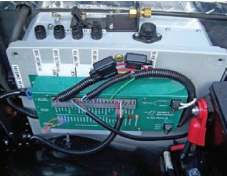
The control box, with the logic interface mounted on its cover.
