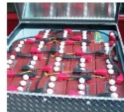
Eighteen of the original FLA batteries in a custom-built box in the truck bed. The six other batteries were housed under the truck's hood.
